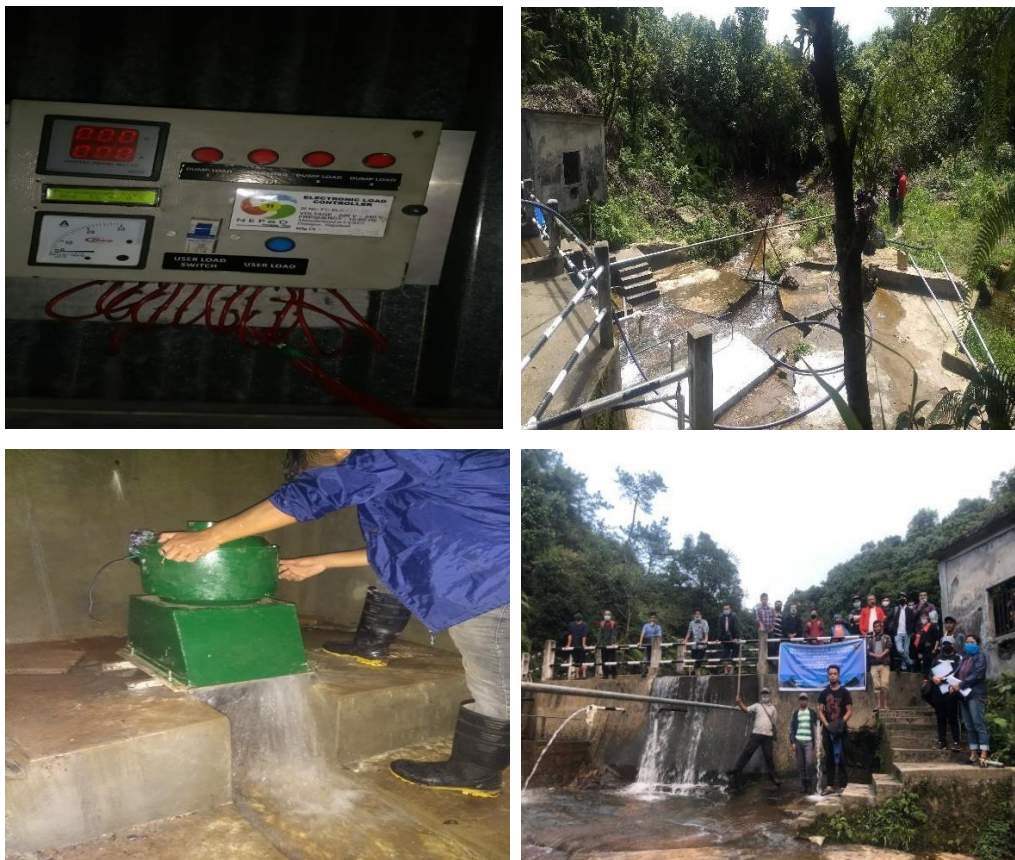
SITE INSTALLATION PICTURES
