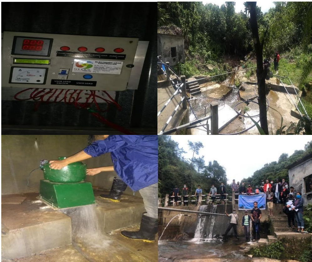
SITE INSTALLATION PICTURES
