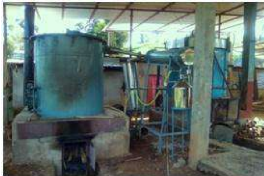
Figure 4: Improved Field Distillation Unit installed at Farmers Field
